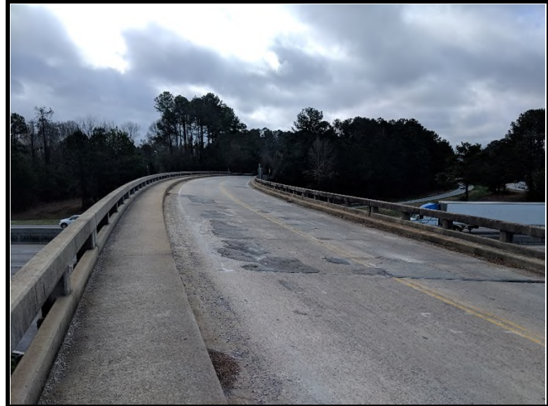
6 No scuppers were observed during the assessment of the bridge.
