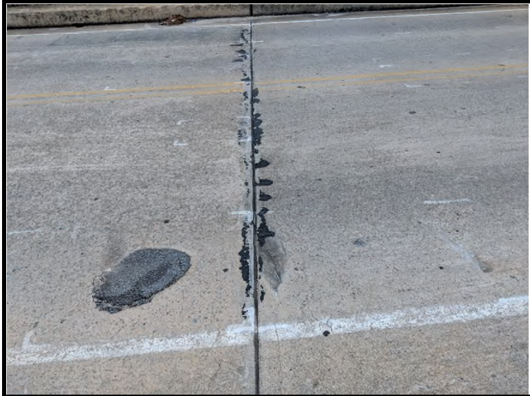
5 The expansion joint material tested negative for asbestos via PLM and TEM analysis.
