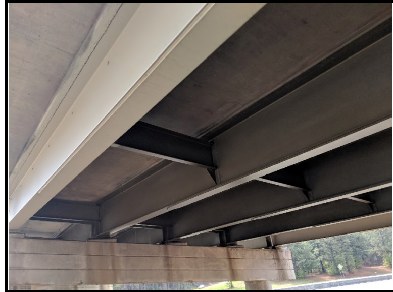
4 View of bent caps. The vibration dampeners tested negative for asbestos via PLM and TEM analysis.
